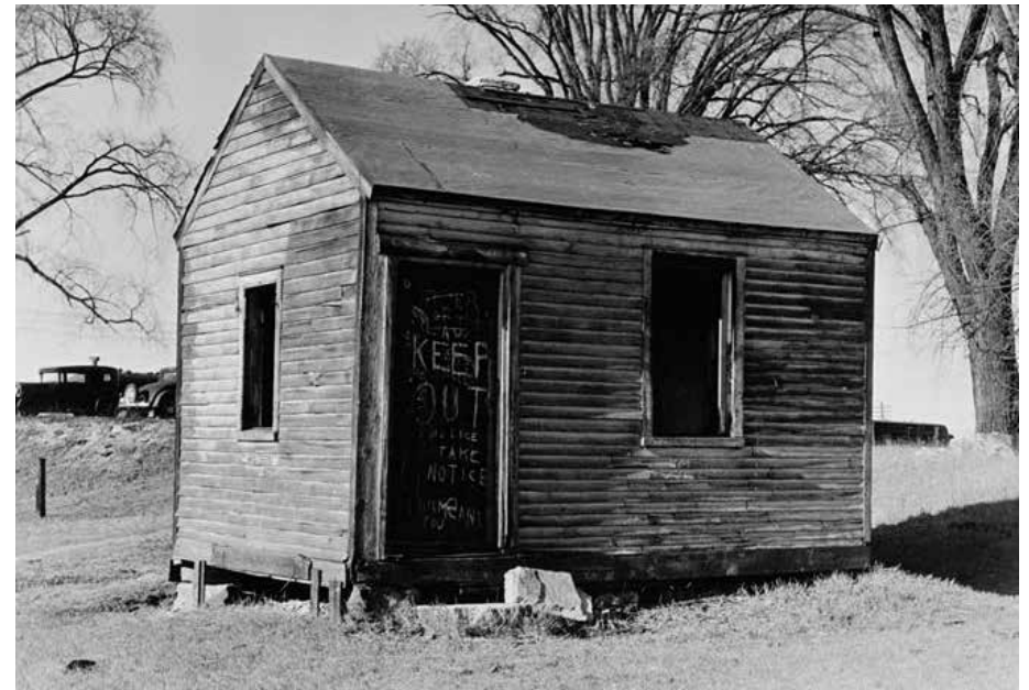
The long-abandoned tollhouse at the top of the Merrimack Flight of locks
