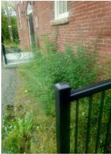
A close up of the weeds around the building in August 2026.
